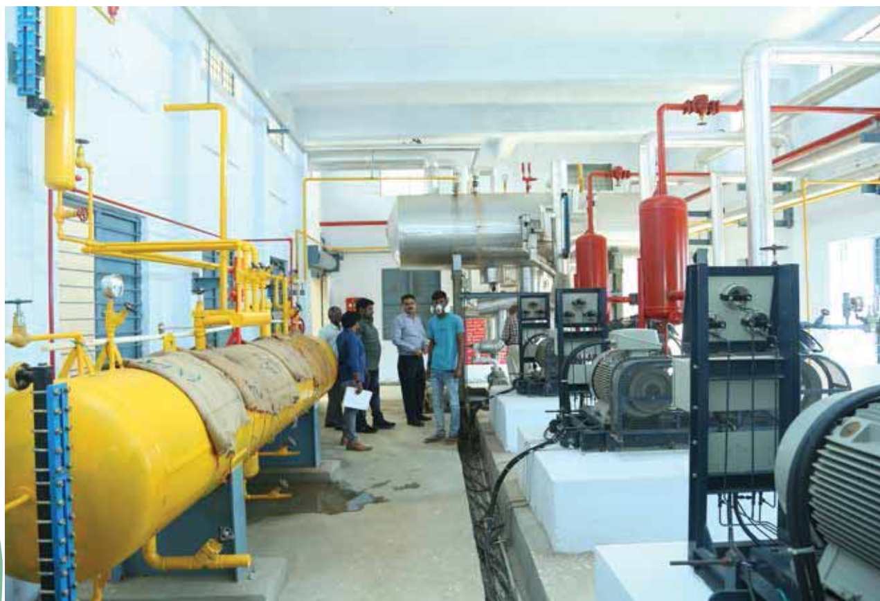
NHB assisted Cold Storage project at Telangana
